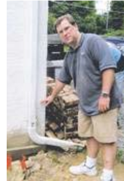
Photo by Amber Healy/The Connection Scott Call, a member of the Acacia Masonic Temple in Clifton, points out how high water from Popes Head Creek rose on the outside of the temple, which suffered some flood damage on the first floor.
