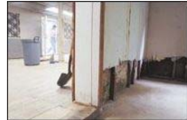
Times Staff Photo/Brian Price Among the destruction from recent heavy storms was the more than 100-year-old Masonic Temple in Clifton. A section of wall had to be cut out, and three floors had to be removed down to the original level.
